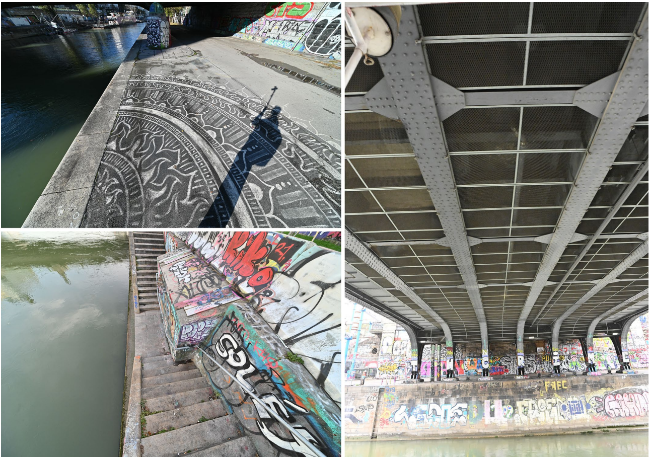
Figure 11 – Two new types of photographs were acquired during INDIGO's total coverage survey. On the left are two photos shot with the camera and a 10 mm wide-angle lens fixed to a hand-held photographic pole. On the right is a photo acquired with the standard 20 mm lens during a touristic boat trip on the Donaukanal.
